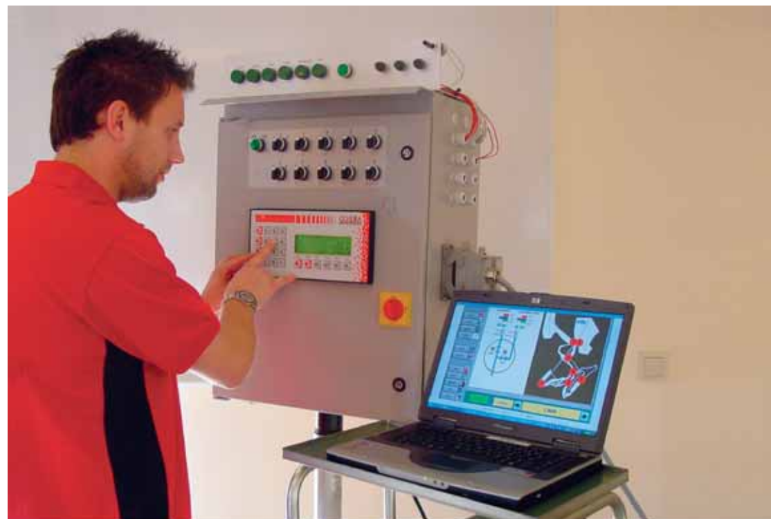
Design Engineer Lars Wärmefors ( ARECO Snowsystem ) is tuning the automation units of the snowmaking system
